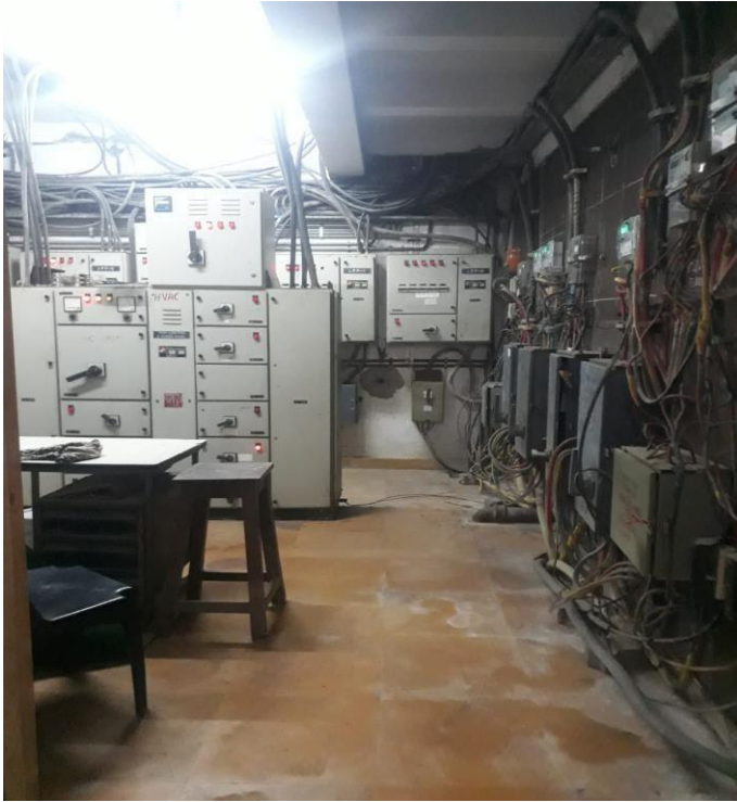
• Electrical Room in the College
