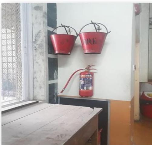
Fig-1. Fire Extinguisher on each Floor
