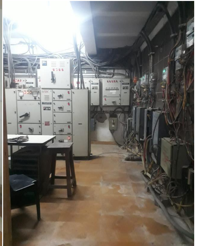
• Electrical room in the college
