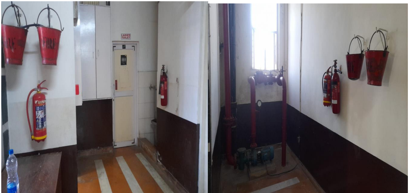
Fire Extinguishers &amp; Sand Buckets at TSEC
