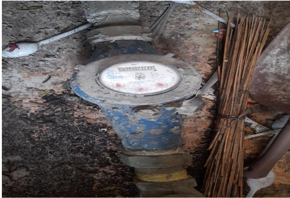
Water Meter 8911190, size 40mm
