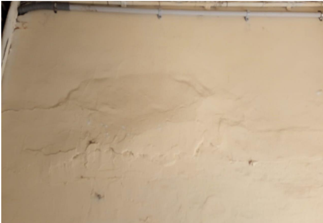
Old building seepage (First Floor)
