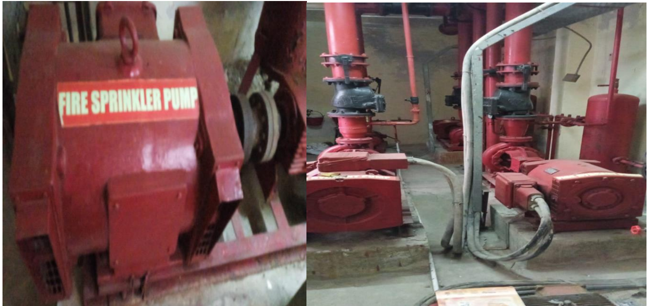
Fire Hydrant and Pumps (NB Ground Floor) at TSEC
