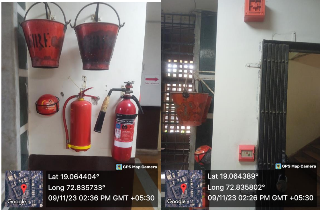
Firefighting Equipment in the New building
