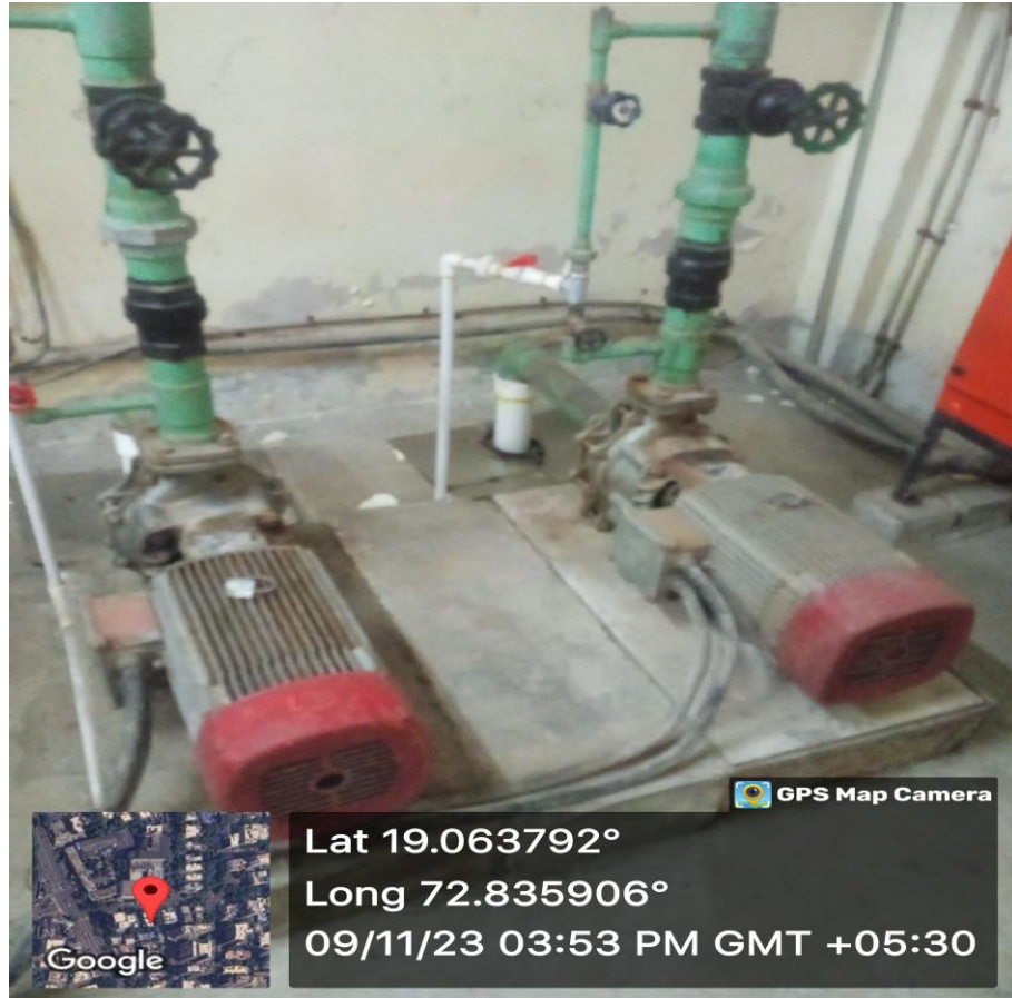
Drinking Water Pumping System
